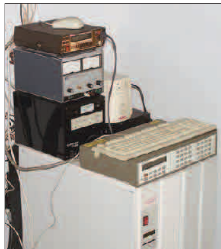
The “home side” of WA2IKL’s PriUPS power system. To get the full story, see Richard’s Web site at www.priups.com/ .
