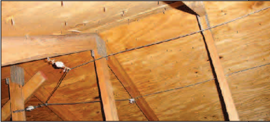
Figure 2 — The inverted L element is supported by egg insulators suspended from the rafters in the attic.
