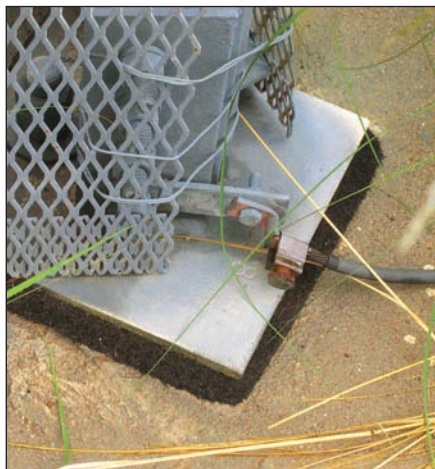
Figure 2 — Tower leg grounding pigtail attachment. All hardware must be rated for dissimilar metal application. Ox-Gard is applied to the exposed copper wire connections every two years to minimize oxidation.
