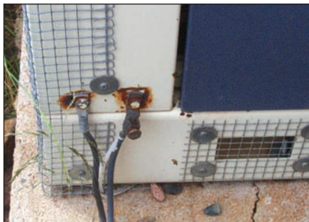
Figure 3 — The generator grounding point after a few years of service. These connections have since been cleaned with a wire brush drill attachment, reattached and painted to reduce future corrosion.
