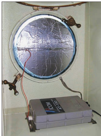
Figure 2 — Inside capacitor plate and connections to AT-130 tuner. Note ground connection.
