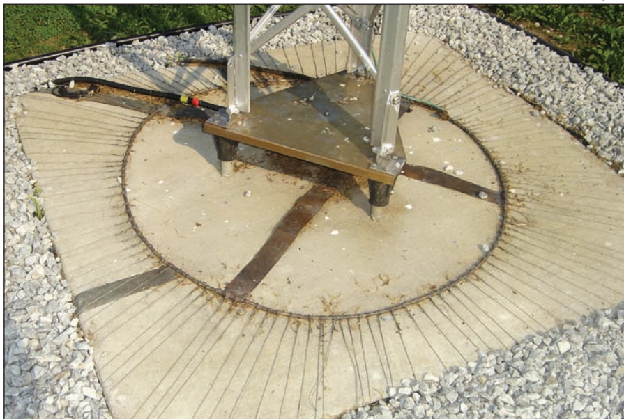
Figure 2 — The station's precise engineering is evident around the base of one of the eight elements that make up the dual K3LR 80 meter phased 4-square vertical arrays.
