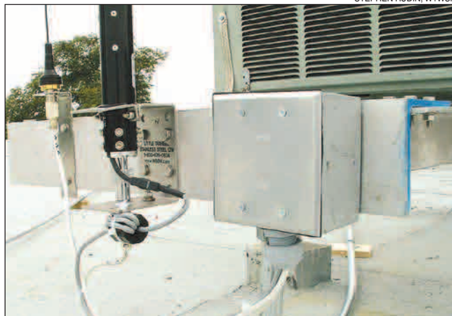
Figure 2 — Close-up of the antenna mounts, cables and the ferrite choke on the antenna control cable.
