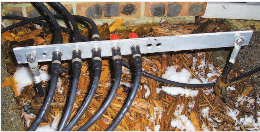
Figure 3 — The outside grounding bulkhead.
