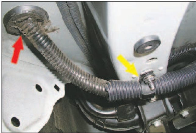
Figure 3 — The dc power cable entering the luggage compartment. The red arrow points to the sealed rubber hole plug. The yellow arrow points to a cable clamp attached to an exposed screw shaft.
