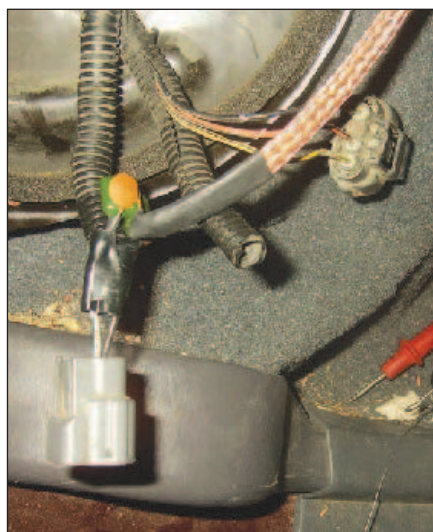
Figure 7 — Details of fuel pump connections ready for bypass capacitors. This is accessible via a small port under the rear seat.
