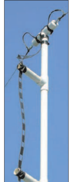
Figure 6 — A close-up view of the mast head and the stand-offs.
