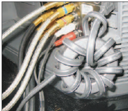
Figure 2 — A common mode choke on the power line, right at the receiver, attenuates RF on that path.
