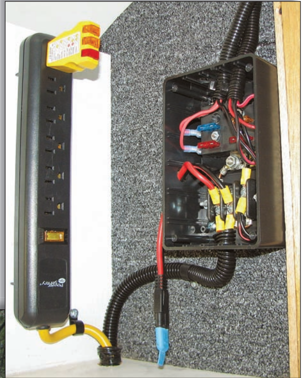
Figure 2 — The 115 V ac “shore-power” outlet strip and 12 V dc fuse/distribution box installed in the Teardrop’s cabin.
