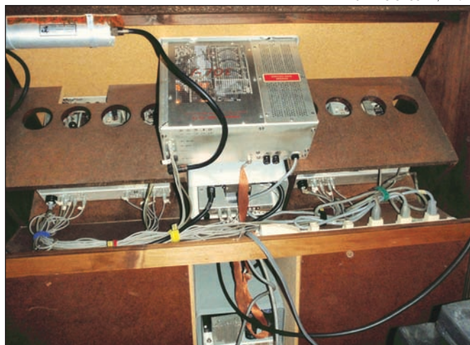
Rear view showing cable layout.
