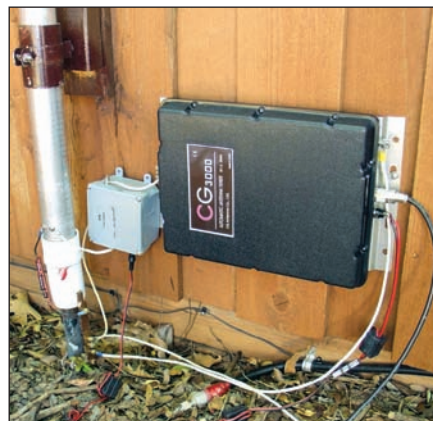
Figure 10 — The ATD-1 mounted with an autotuner at the base of the author's 43 foot vertical antenna.
