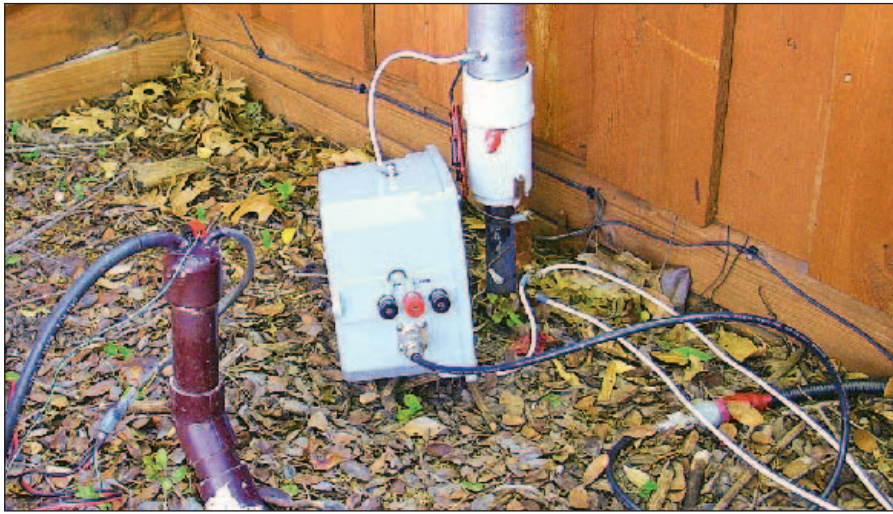
Figure 7 — Matching unit at the base of the author's 43 foot antenna. In this view, it is strapped for 80 meters.
