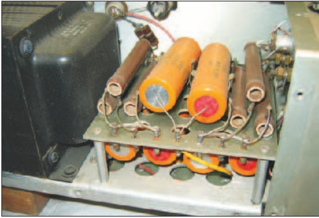
Figure 3 — The original filter-bleeder board (on posts) and the rectifier board (below the chassis) before replacement.
