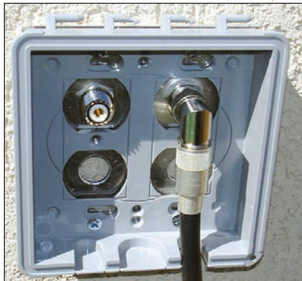
Figure 3 — The assembled and mounted outlet box containing two UHF connectors. A neat and tidy installation.
