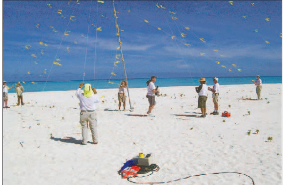
The K4M team installing one of the low band verticals on the beach. The yellow flags on the guys and vertical were a requirement of the USFWS so the local birds would not fly into them.
