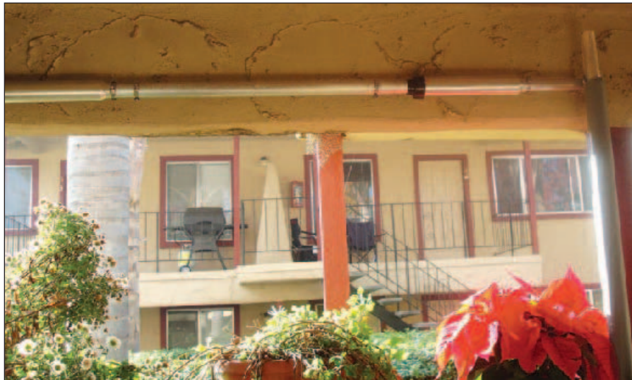
Figure 2 — The horizontally mounted portion of the antenna, as seen from inside the patio.
