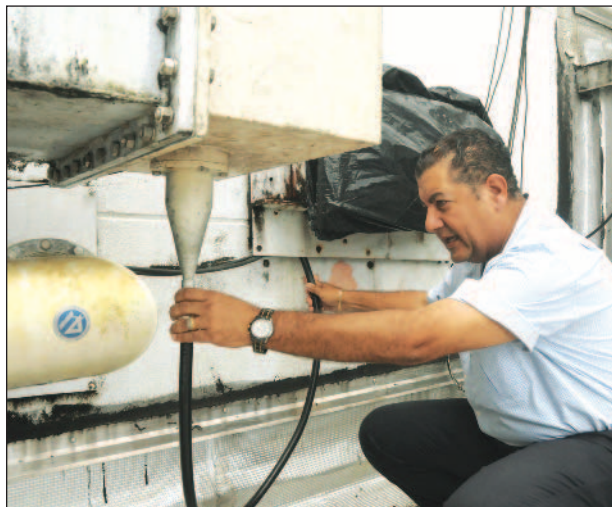
Angel, WP3R, connects LMR-900 feed line to a waveguide-to-coax transition, just outside the transmitter room.
