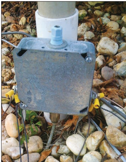
Figure 3 — The hardware store electrical box contains all the interconnections.
