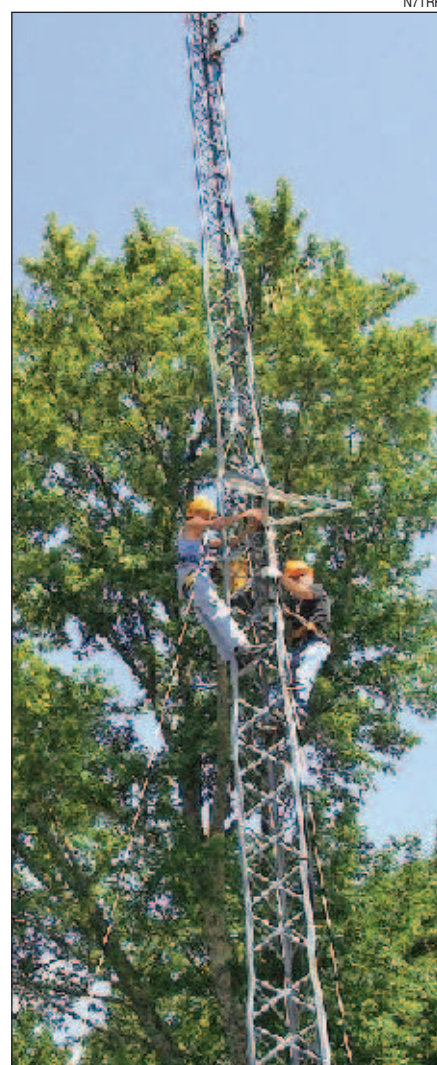
Figure 4 — Panel bracket installation by Al Perkins, KA1KIX, on left, assisted by KT4BW.
