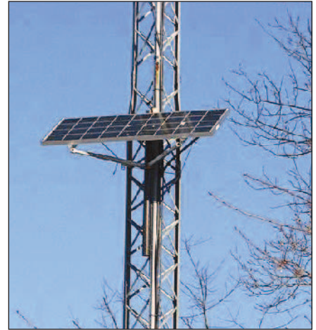
Figure 6 — 130 W PV panel on line in Tennessee.
