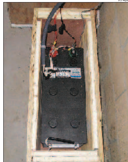
Figure 3 — Selected battery for our system, a Deka 12 V, 198 Ah unit. This battery weighs 130 pounds. Insulated battery box designed and constructed by Joe Koester, W4NSA.
