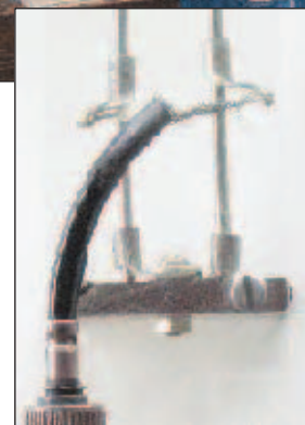
Figure 2 — View of antenna feed connection details.
