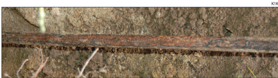
Figure 2 — Guy anchor rod inspection. This rod has lost all of its galvanized coating, exposing the steel to corrosion.
