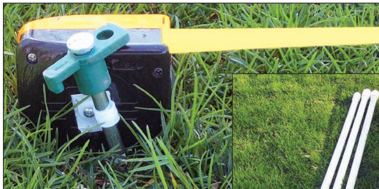
Figure 3 — Staked radial detail. Note \frac{3}{8} inch cable clamp and larger housing screw. The end of the radial does not electrically connect to the stake.
