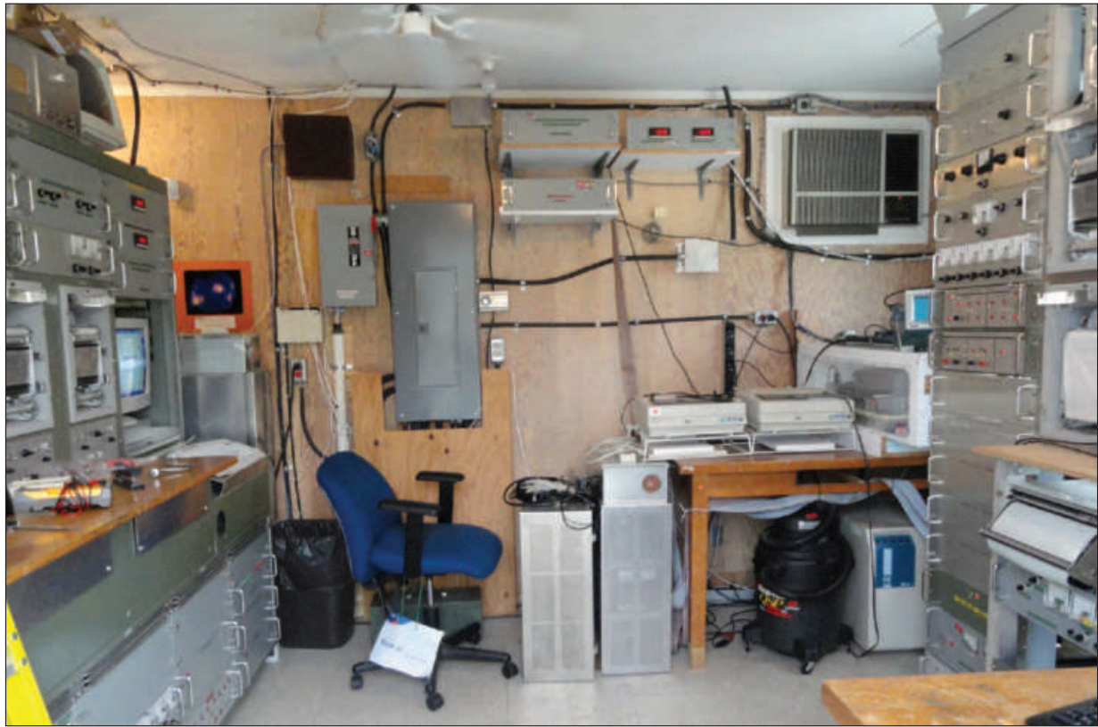
Figure 6 — A view in through the door of the solar hut. The FM1 rack is on the left, and the FM2 rack is on the right.
