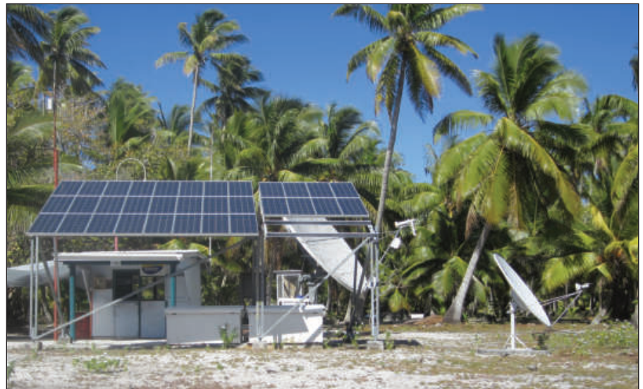
Figure 6 —The solar powered telephone shack provided Internet service within 15 feet and mobile phone service within 100-200 feet.
