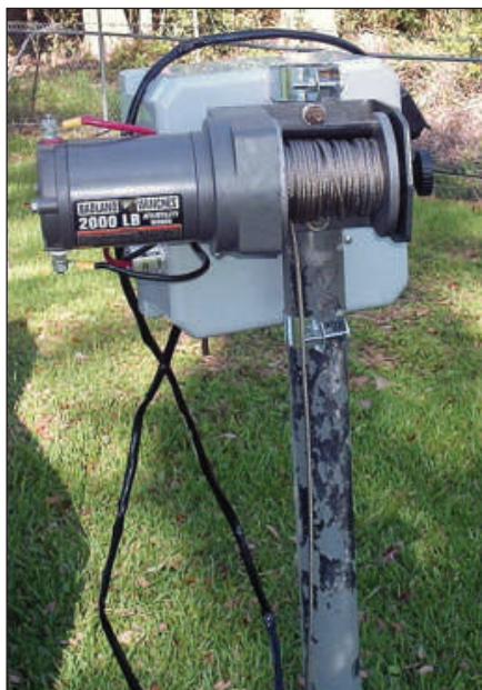
Figure 1 — The winch and control box mounted on the post about 15 feet from the tower. The steel cable runs down to a pulley at the base of the post. [Pat Hamel, W5THT, photo]
