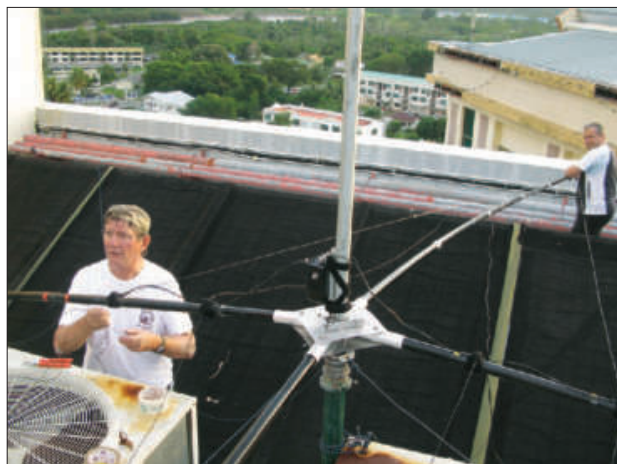
Michel, F5EOT (left), the V84SMD HF “Antenna Magician” and Paolo, IW2ETR, installing one of the Spiderbeams.
