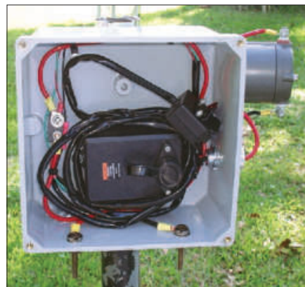
Figure 2 — The interior of the watertight box showing the winch control unit and pendant in their storage locations. At the bottom are the two brass screws used as 12 V connection points. [Pat Hamel, W5THT, photo]
