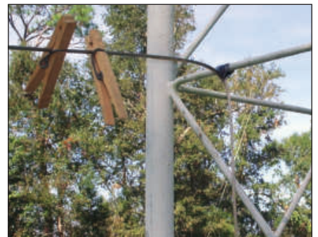
Figure 4 — The cable, in “clothesline mode,” is taped to the tower about 6 feet up. [Pat Hamel, W5THT, photo]
