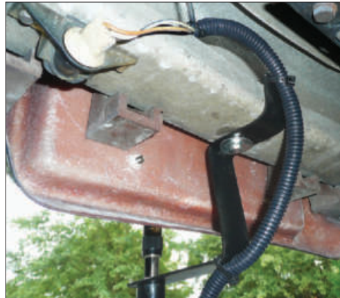
A close-up view of the antenna mount where it attaches to the frame.
