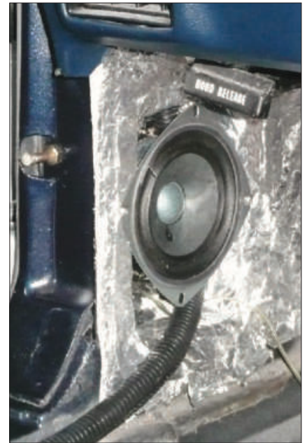
Here is one of the transceiver's external speakers being installed behind a kick panel.
