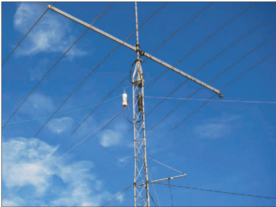
Figure 6 — Balun and antenna mounted on tower.
