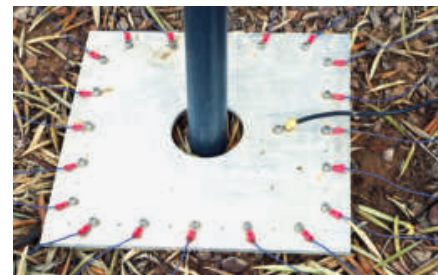
Figure 3 — A square aluminum plate is drilled and tapped for 40 radials. The black wire is the ground connection for the MFJ tuner. [John Marshall, WA7BSR, photo]
