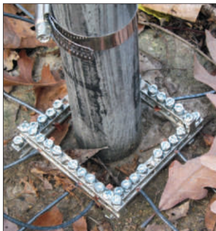
Figure 7 — A set of four equipment grounding bars can be bolted together to form a square around the base of your antenna and they will provide ample connection points for radials. [Richard Steck, W9RS, photo]
