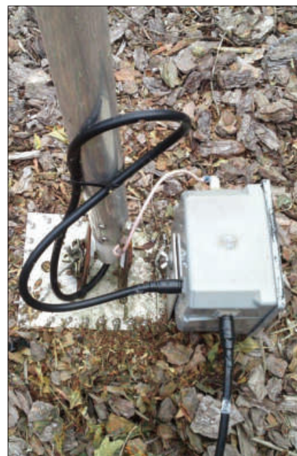
Figure 2 — The 43 foot vertical antenna attached to its insulated swivel base. The dipole's coax feed enters through the hollow Delrin rod that forms the base insulator. The gray electrical box contains an MFJ 10-10989D wired as a 1:4 unun.
