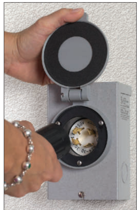
Figure 5 — An outdoor twist lock connector for generator connection. See the sidebar entitled "The Generator Connection" for more information.
