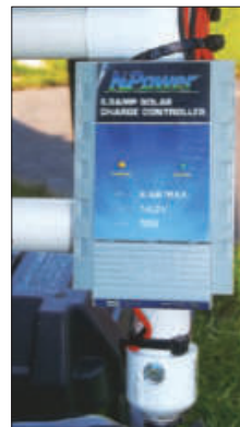
An 8.5 A solar charge controller installed below the solar panel.
