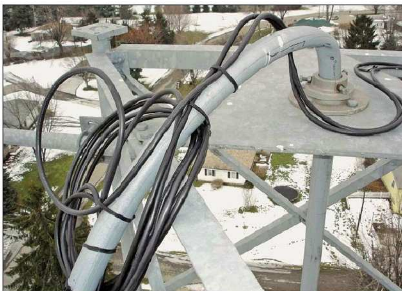
Figure 1 — A water pipe mast failure. [Thomas Cox, KT9OM, photo]
