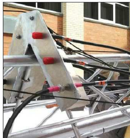
Figure 7 — Mounted just below the top of the tower with U-bolts, the coax connector plate provides a convenient transition place to change from stiff to flexible types of coax. [Dennis Klipa, N8ERF, photo]
