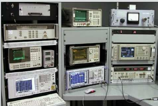
A view inside the screen room. The new Agilent MXA-9020A spectrum analyzer is visible at the lower left and the new Rohde & Schwarz FSUP 26 signal analyzer is at the bottom of the center rack.
