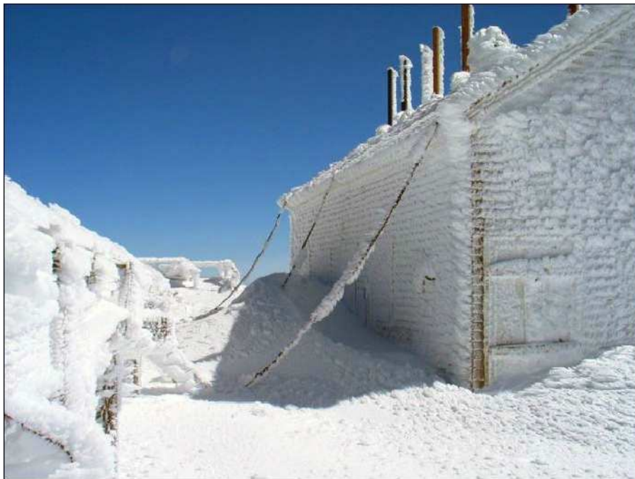
In blizzard conditions, anchoring tents and even small structures is critical. This anchored building is at the summit of Mt Washington. [NOAA photo]
