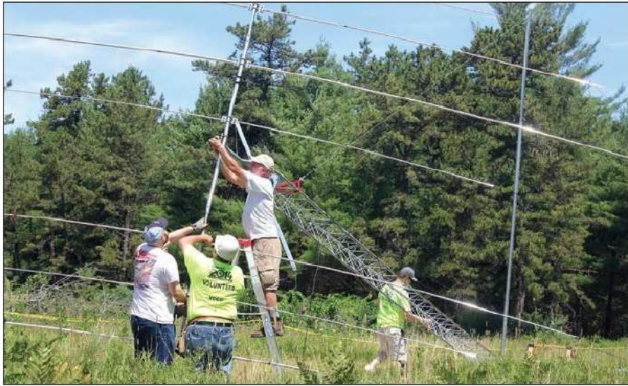
A beam team installs the tribander on the tower [Marian Deacutis, KB1YLJ, photo]
