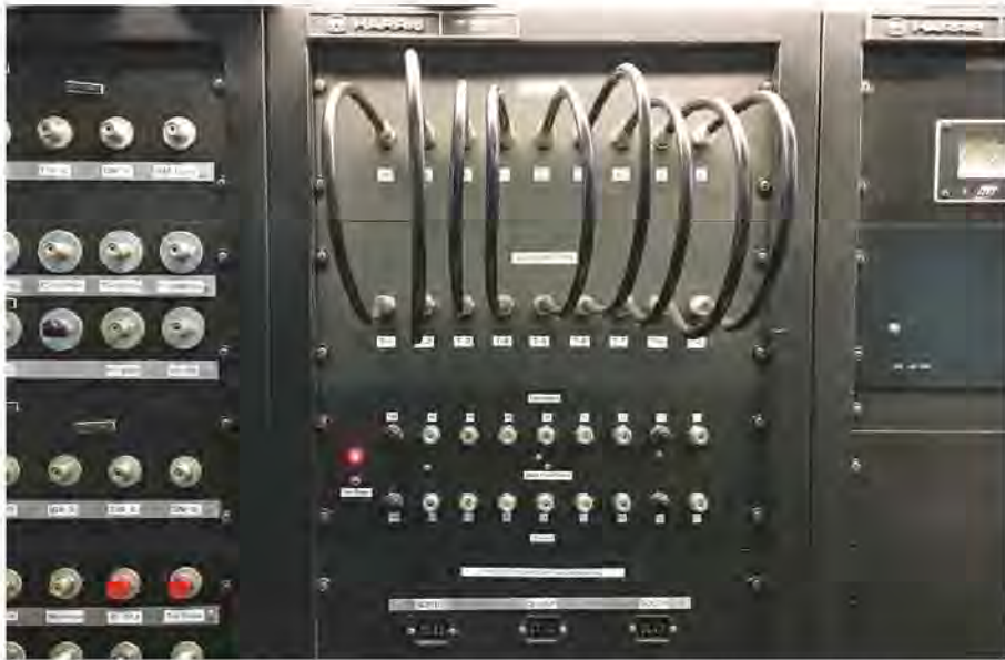
Figure 2 — View of a portion of the W1AW patch panel used to interconnect transmitters and antennas using coax jumper cables. Yours probably doesn't need to be quite as extensive [Joe Garcia, NJ1Q, photo].
