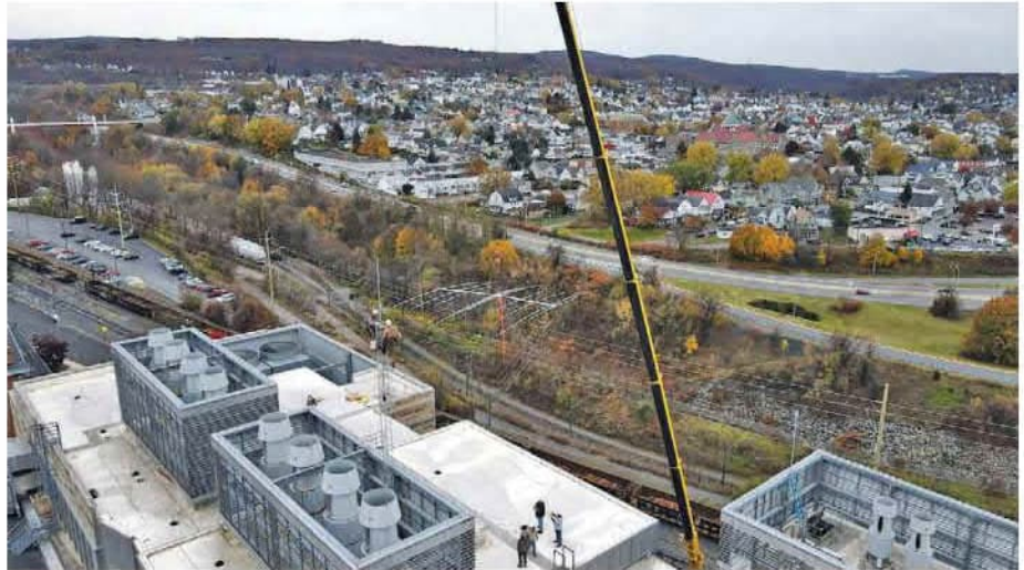
A crane lifts an antenna into place for W3USR's new location. [Byron Maldonado photo]
