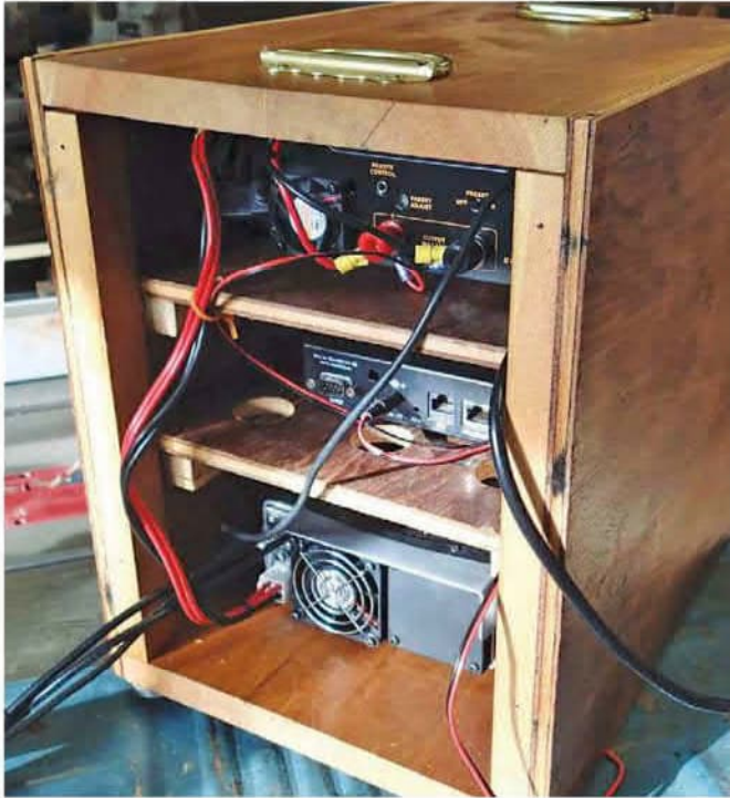
The back of the station in a box as it was being wired.
