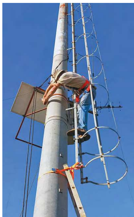
Olaf Bucking, V51OB, works on the tower to secure the antenna feed line. [Namibian Amateur Radio League photo]
