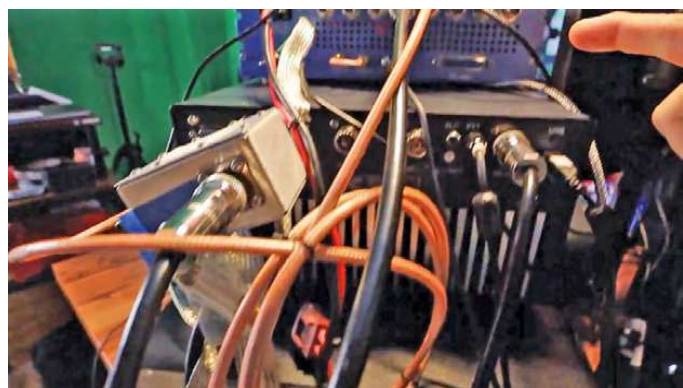
Darren, N4VFR, shows viewers the cables at the back of his operating position, which he works with to attempt to eliminate the RFI problem.
