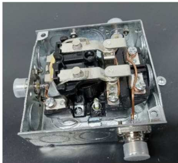
Figure 3 — Mounting of the relay and the SPDT wiring. [Robert J. Zavrel, W7SX, photo]
