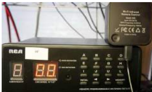
Figure 2 — The Wi-Fi infrared hub shown atop the RCA VH226E controller. [Tommy Walls, KC4ZZE, photo]
