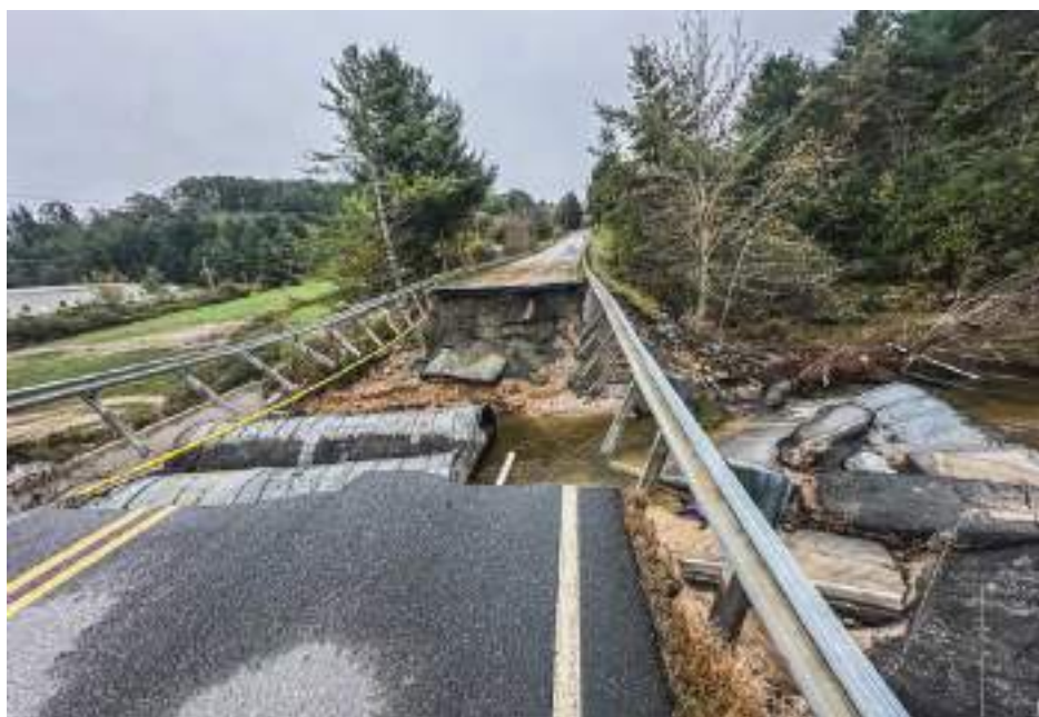
A roadway in North Carolina destroyed by Hurricane Helene. [US Customs and Border Protection Special Response Team photo]
