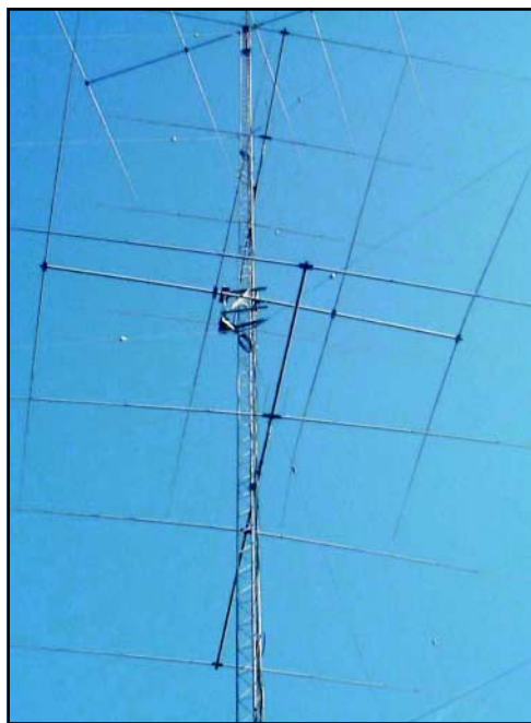
The swinging gate mount and Yagi (middle portion of photo) completely installed on the tower.
