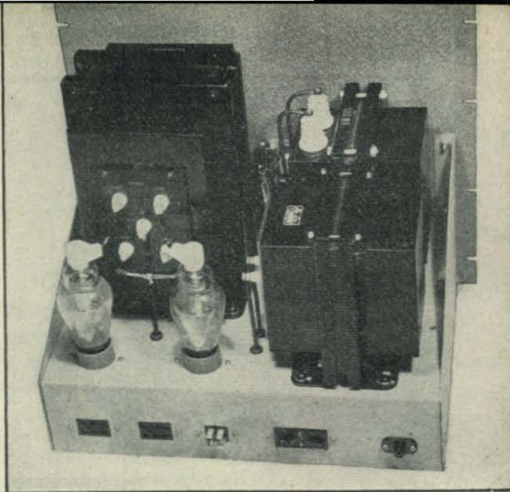
750 watt supply. Note the safety connector for HV, safety caps on the rectifiers, and 20 amp circuit overload relay which protects the entire transmitter. Safety sockets for the 866A's are added insurance against voltage breakdown
