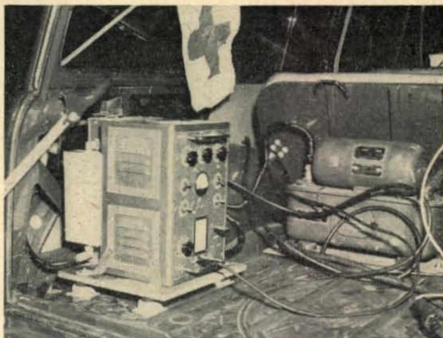
Side view of Harvey-Wells TBS-50 installed in Plymouth station wagon, showing copper screening over louvres.
