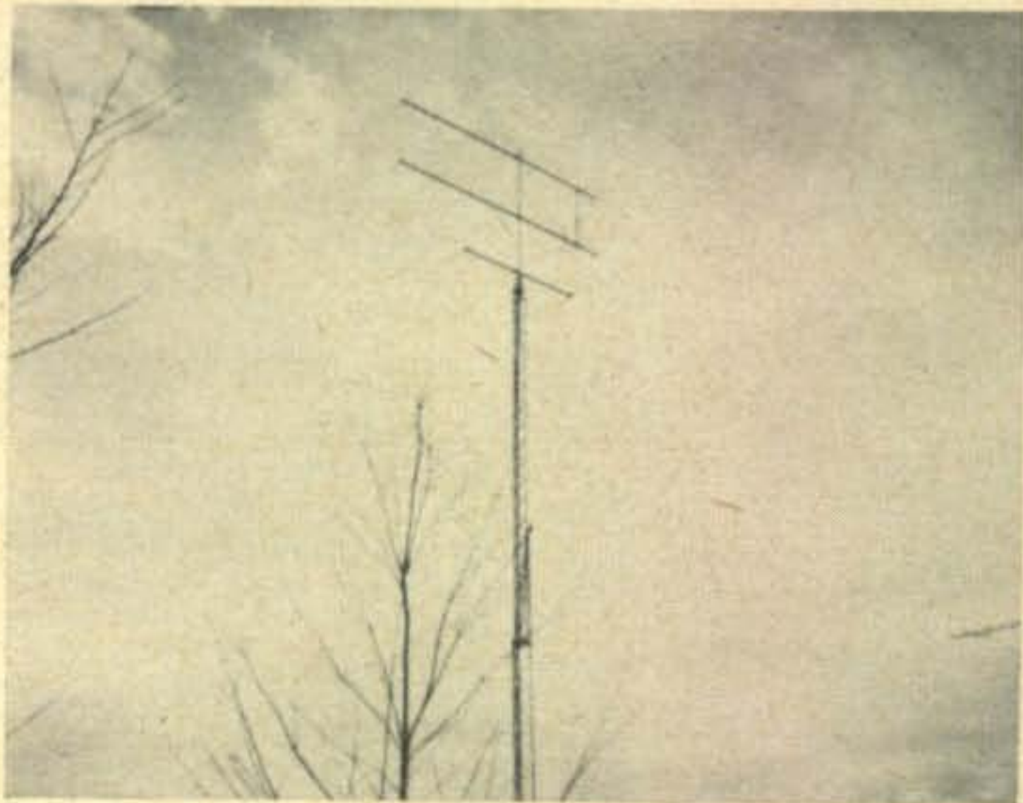
60 feet of Elprodco with 20 feet of mast extension. 8X8 Telerex on Two and 3 element Telerex on Six at WØUSQ
