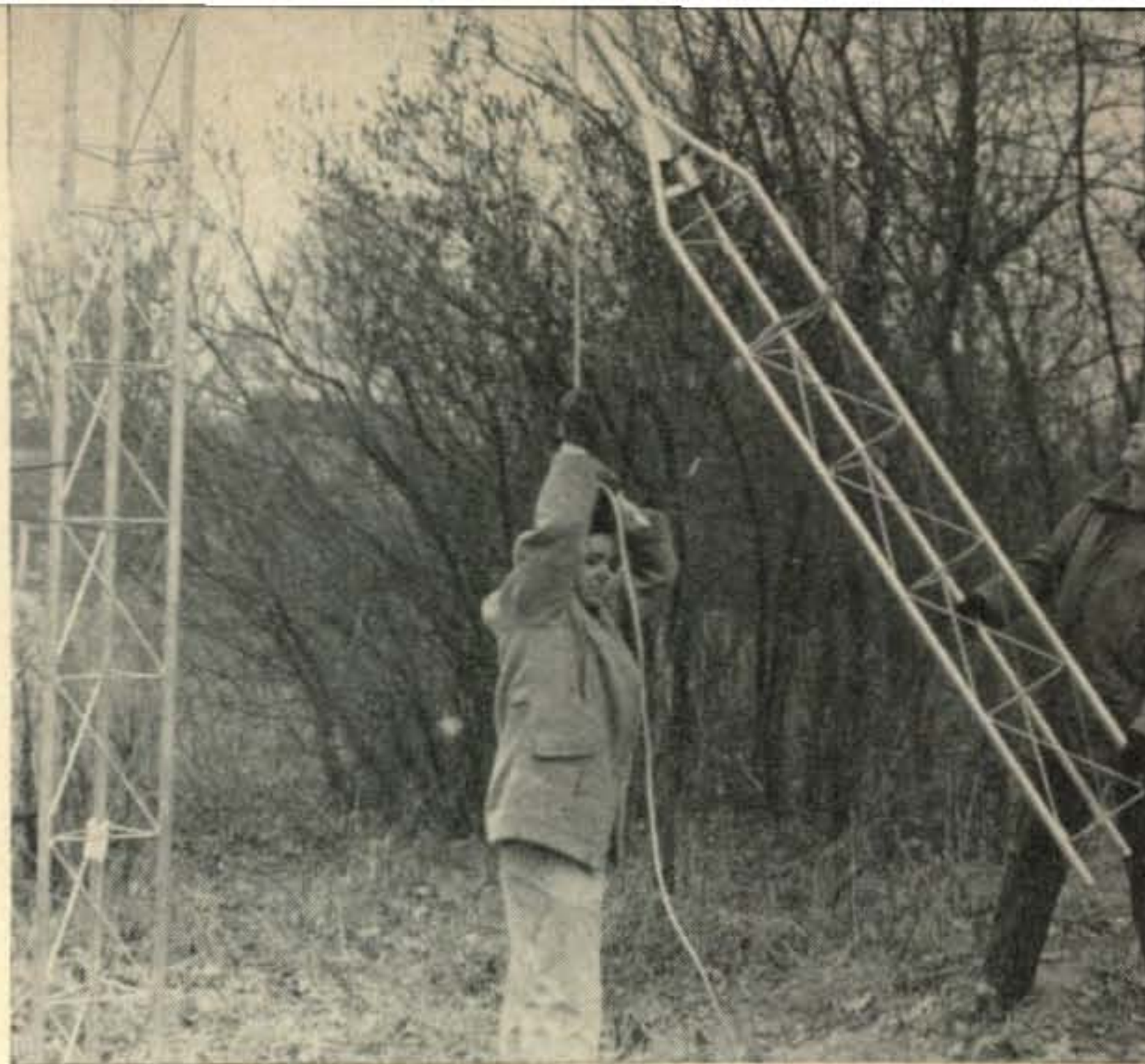
UP She goes! Top section of W1FRR's new 110 foot high tower (Rohn) being sped on its way by Fred (W1FRR) and Paul (W1PYM).
