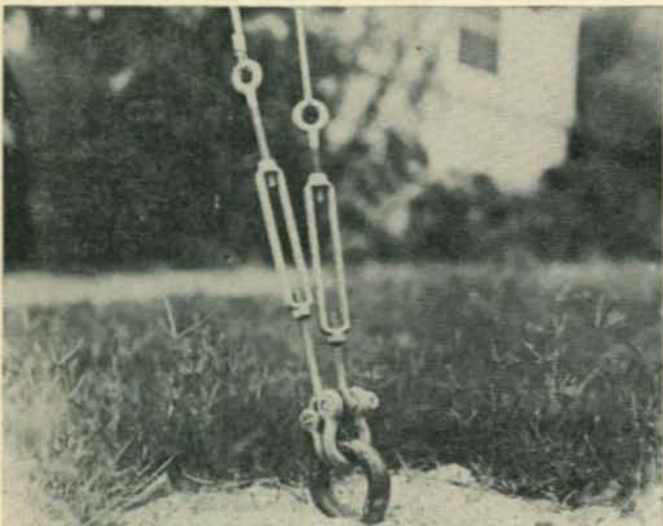
Fig. 8—View of the upper and lower back stays secured to the anchor bolt with shackles. Number 6 Burndy electrical clamps are used to secure the wire.
