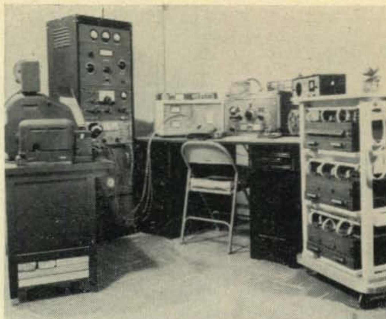
Overall view of the station. The printer is on the left of the rack containing the transmitter and TU. The control panel for semi-automatic operation is on the left end of the operating desk. The multi-gate units are racked up to the right of the desk.
