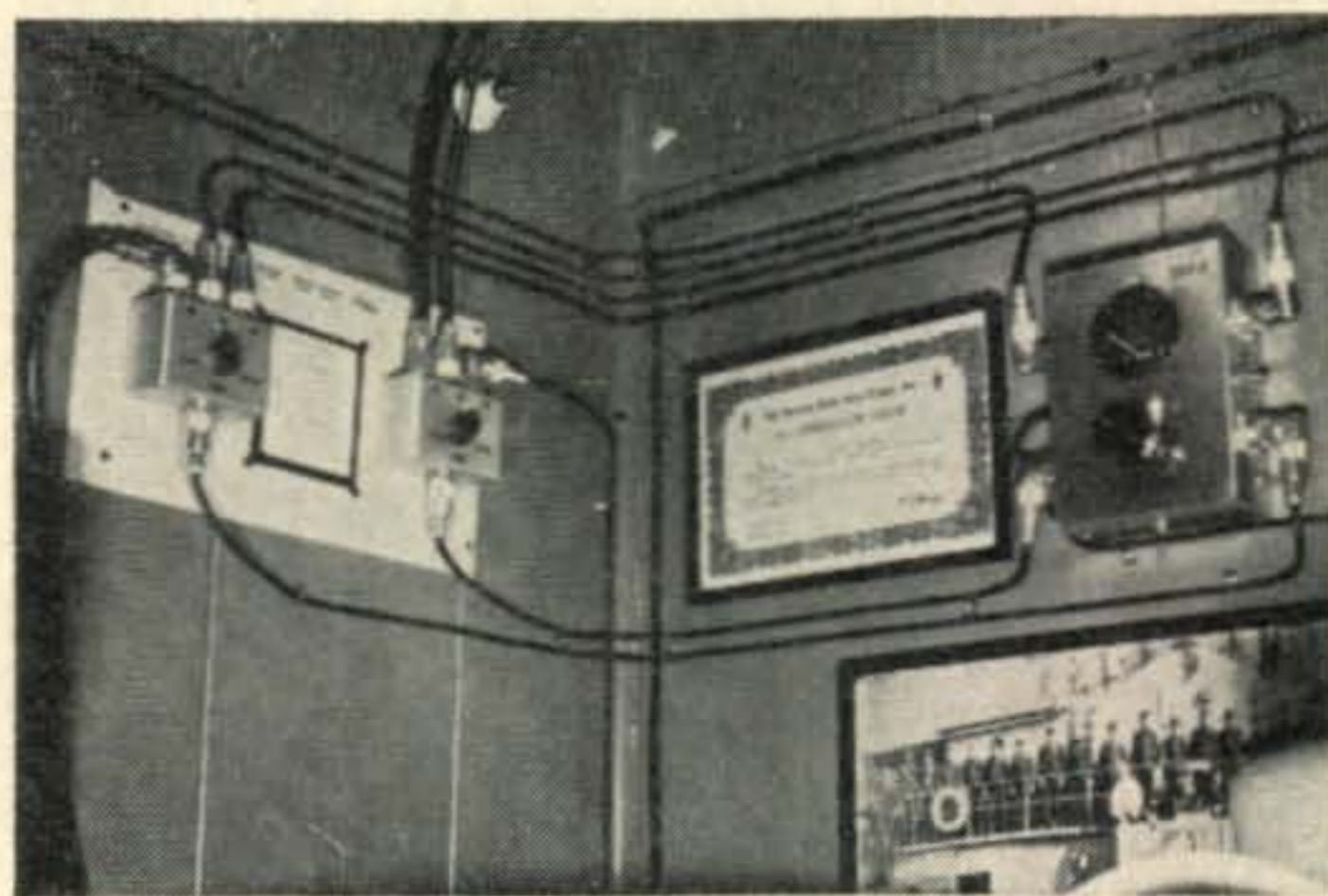
The transmitter/antenna panel and antenna group selector unit installed at W7OE. The transmitters are located below the panel and an identical receiver panel is located at the opposite end of the shack.
