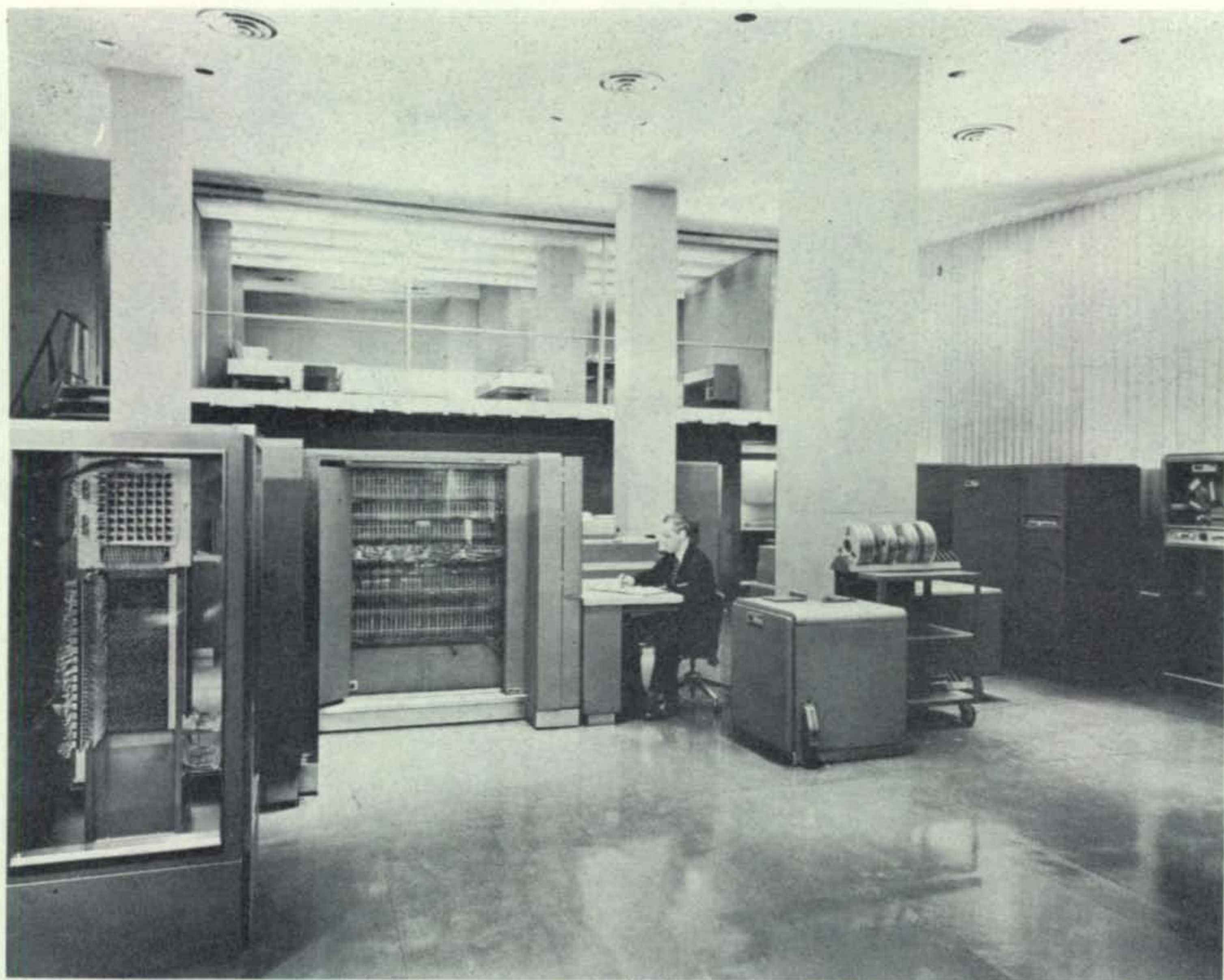
Electronic data processing equipment such as shown, incorporating thousands of intricate components, offers a wide field of opportunity for skilled electronic engineers and technicians.
