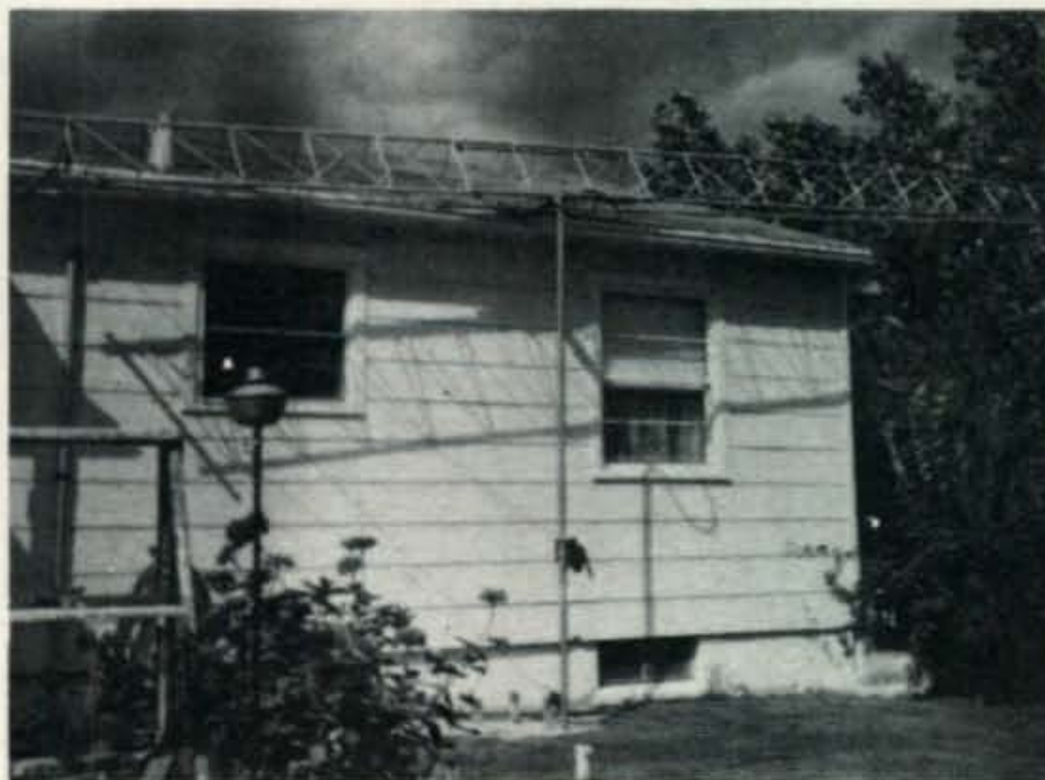
Fig. 2—In the down position the tower is nearly parallel to the roof eaves. The 1 1/4" support pipe extends 10' into the house and is bolted to the joists. The bottom of the pipe is 4' into concrete.
