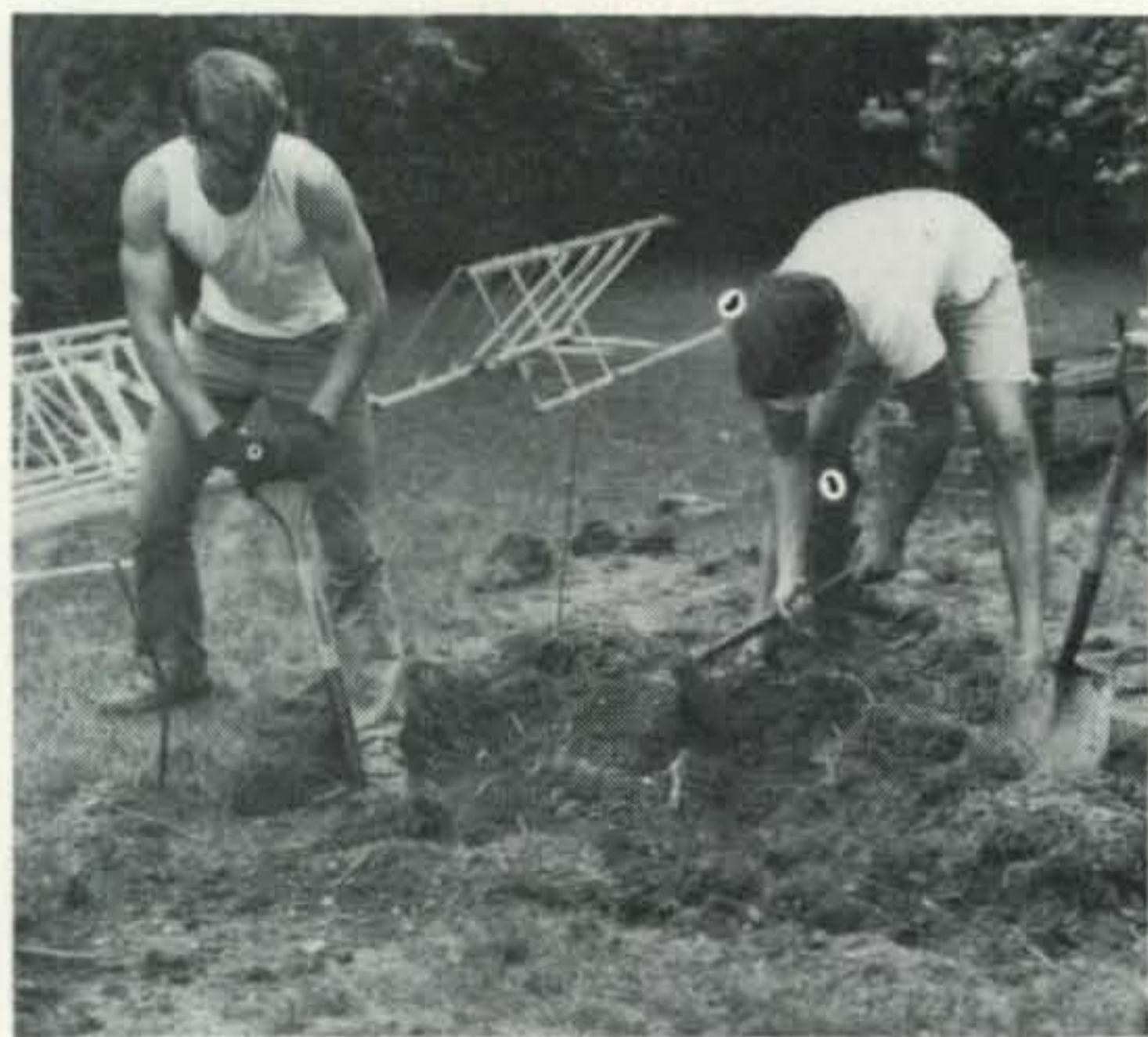
Careful locating of the base and the hole for it are absolute musts, as explained in the text. Two young huskies begin digging. A layer of clay was found right beneath the surface, probably from backfilling when the house was built. Pick was needed to break through it.
