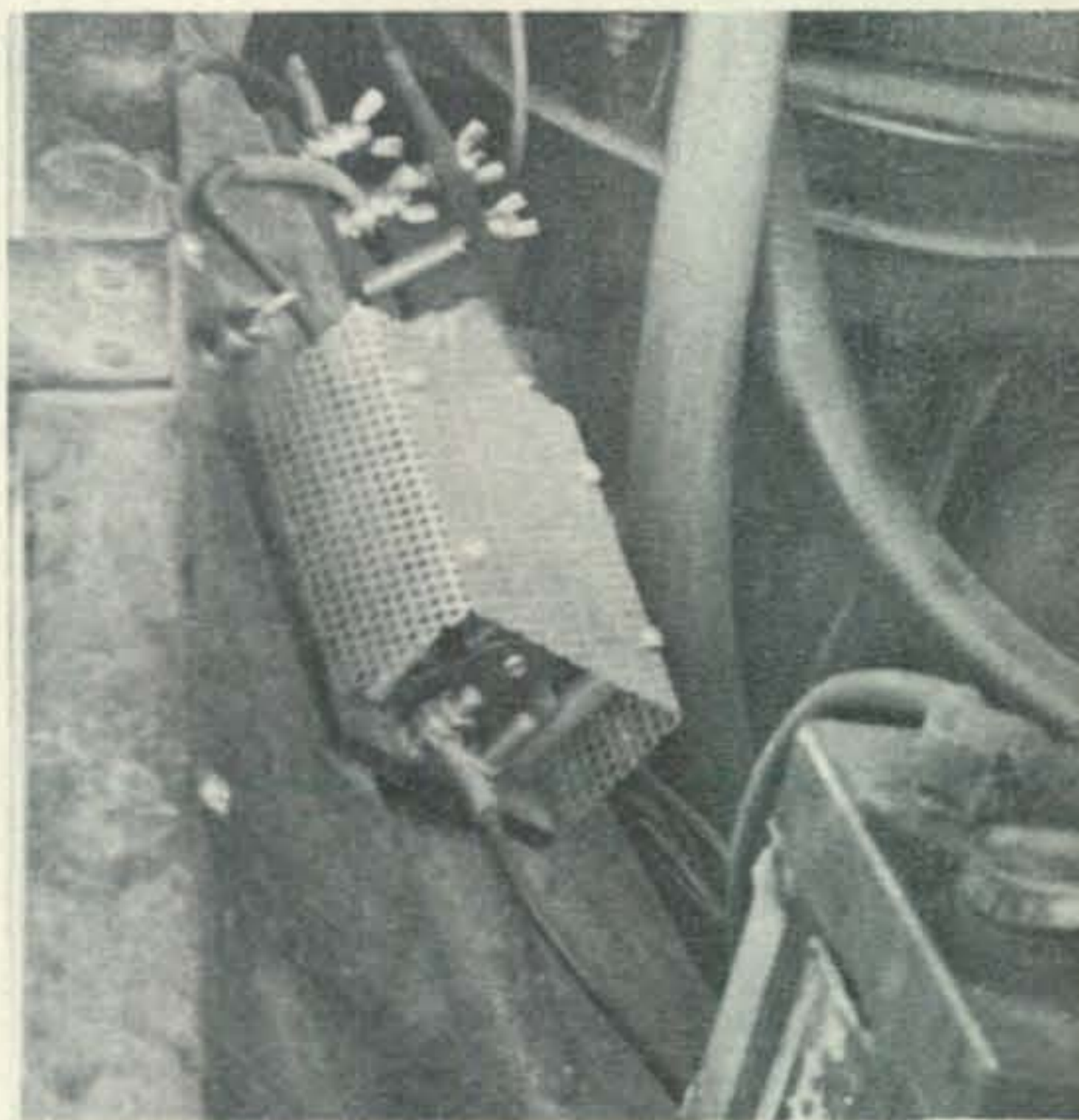
Close-up view of the battery isolating diodes mounted on angle aluminum heat sinks within a perforated cover. Just to the rear of the diode enclosure is the battery disconnect (wing nuts). Both are mounted within the engine compartment of the camper truck on the inner fender well. (Photos by Ted Stites).
