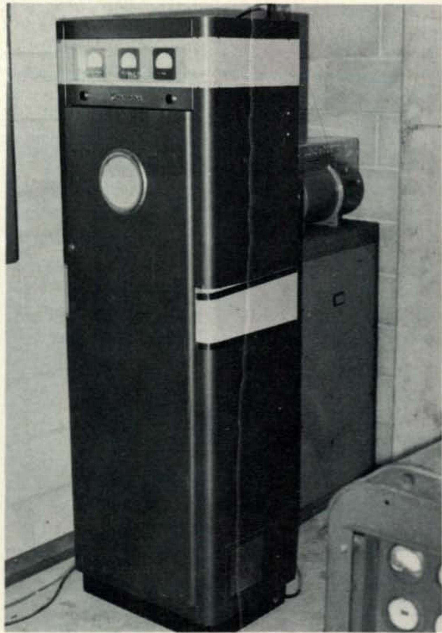
The interior of the emergency generator room atop Stone Mountain near Atlanta, Georgia. The unit is the Atlanta .34/.76 machine.
