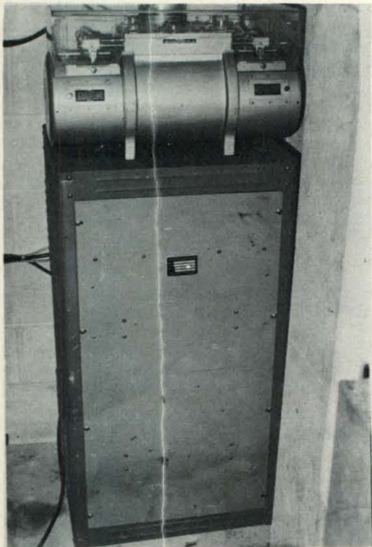
The diplexer for the Atlanta .34/.76 system is on the bottom and the voice id machine is on the top. The unit operates from Stone Mountain Memorial Park near Atlanta.
