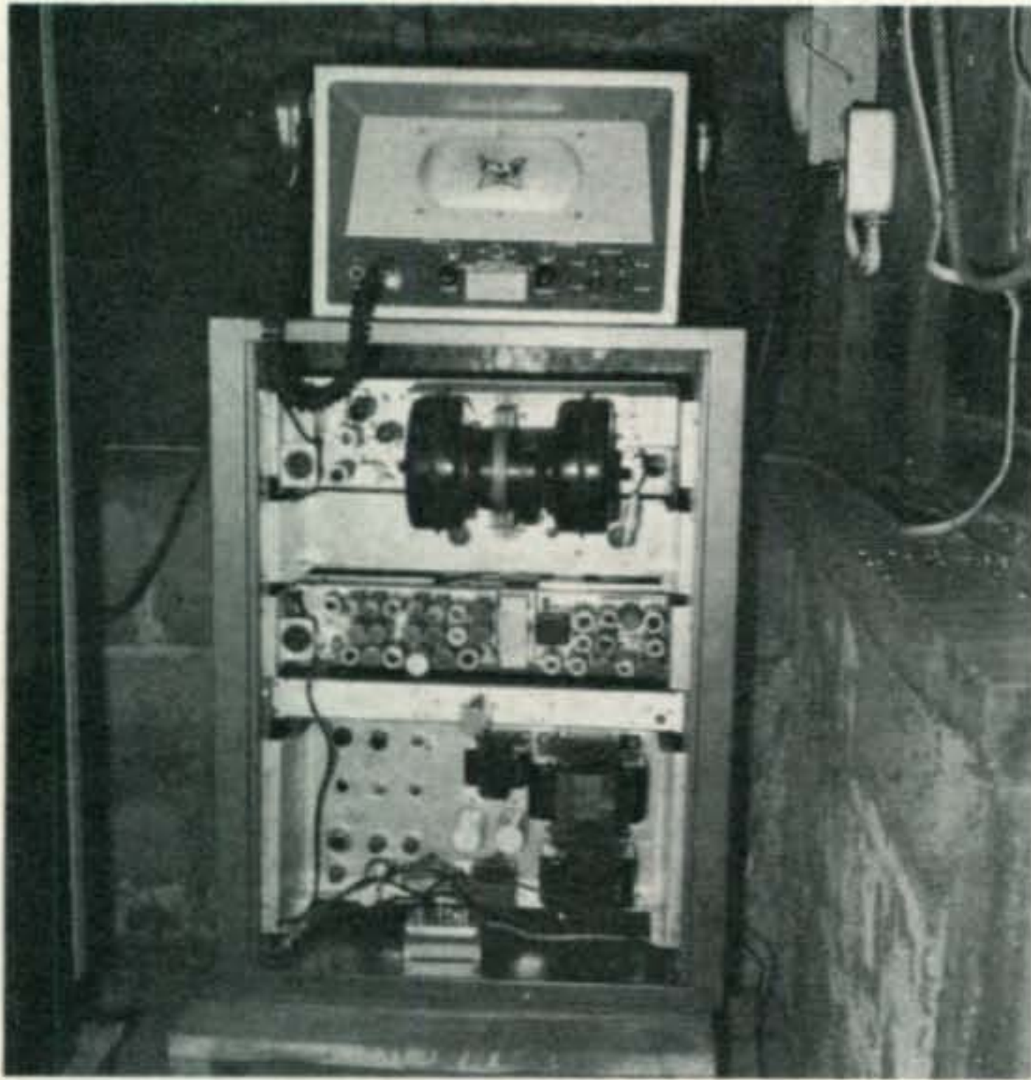
Uplink equipment for the Laurel Mountain repeater. Equipment is RCA.
