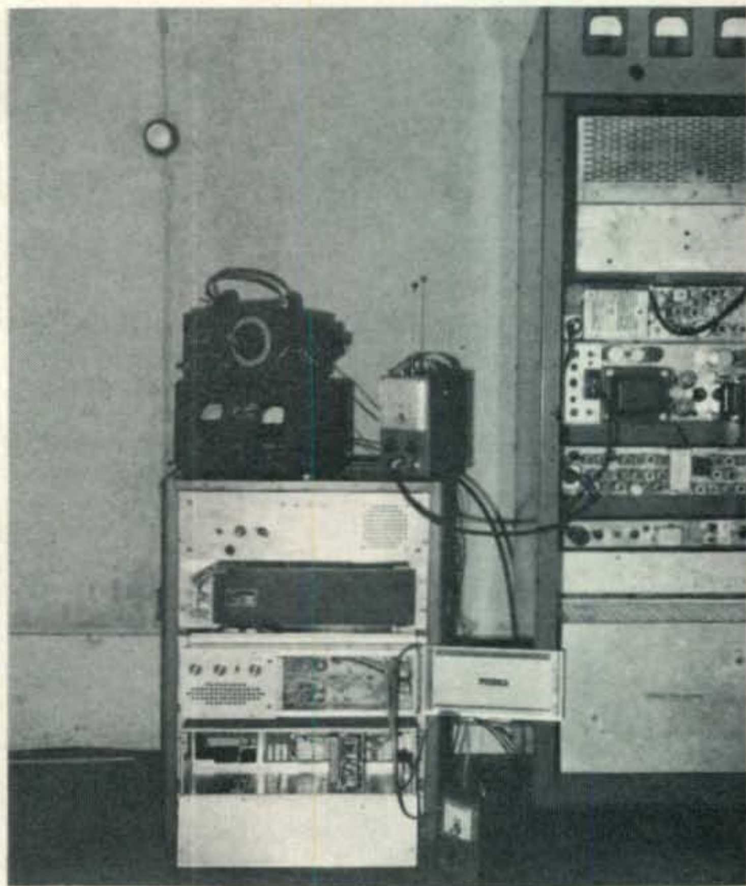
Down link and 146.940 MHz transmitter of Laurel Mountain Repeater. A total of 3 remote 146.340 MHz receivers feed the 250 watt output base. Antenna gain is 5.8 db and location is 2750' above sea level.
