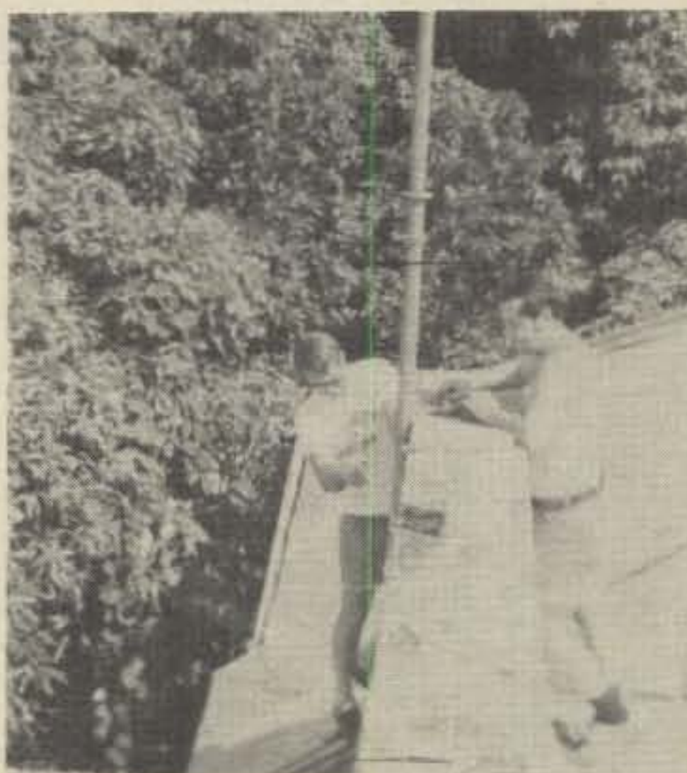
Bill Beggs, N5RR (Left) and Ron Blake, N4KE (Right) install masts atop the Hotel Roi Christophe in Cap Haitien, Haiti in preparation for HH5HR operation in the 1977 CQWW phone contest (NFDXA Photo)
