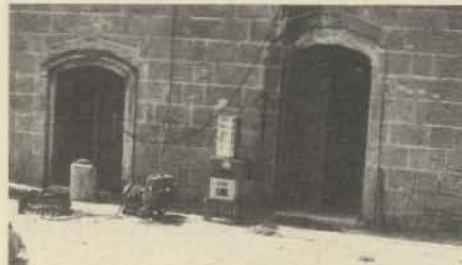
The powerplant of IJ7EX, when the island's main power aggregate was stopped during the night, this little machine was responsible for your midnight QSO.
