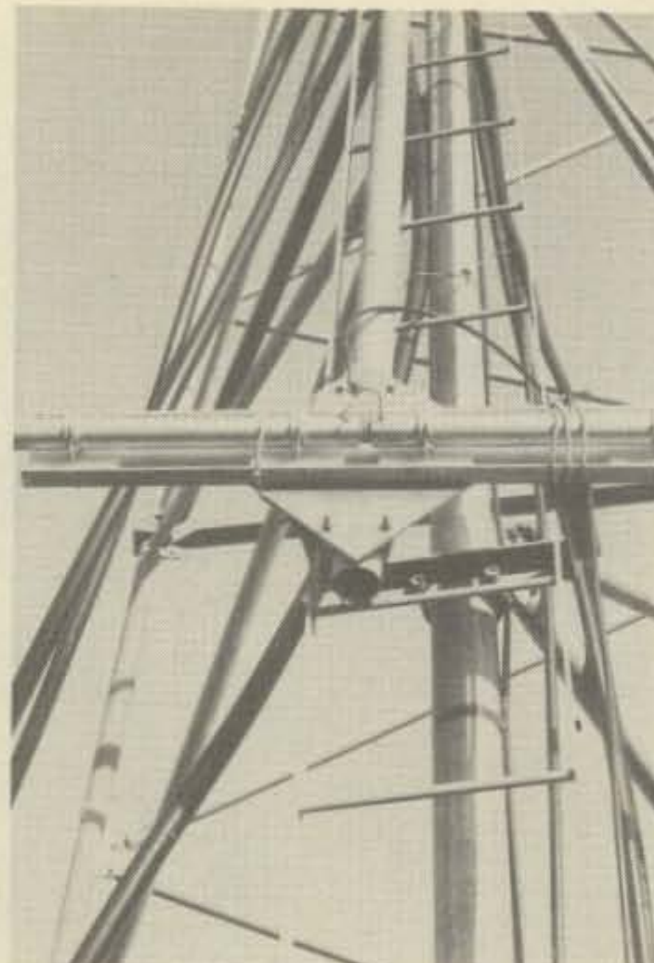
Fig. 8 — The 80 meter beam on its way up the tower, showing the center portion of a driven element. Note the heavy heliax cables coming down the legs of the mast!
