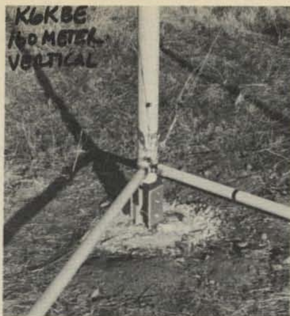
Fig. 12 - The tower at K6KBE is insulated from ground by means of fiberglass plates which hold tower to the mounting base.
