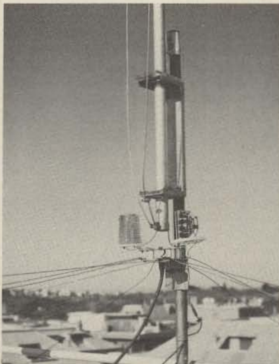
Fig. 4-The base of the I0ZV antenna showing the radial wires, antenna support and 80 meter loading coil. Note the 20 and 10 meter vertical wires running parallel to the aluminum tube.
