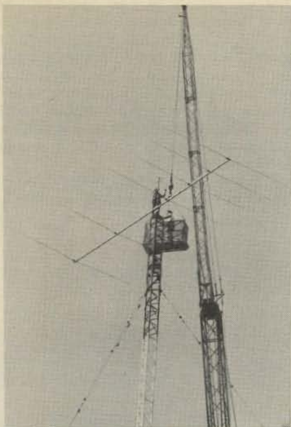
Photo 1 - The 208-foot crane's basket was used to transport the workers to the top of the tower.
