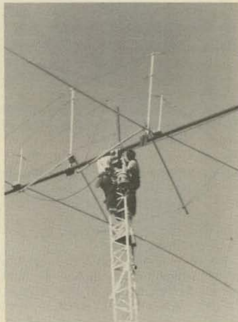
Photo 3 - A sling was placed on the boom and fastened to the horizontal guy lines to maintain stability.
