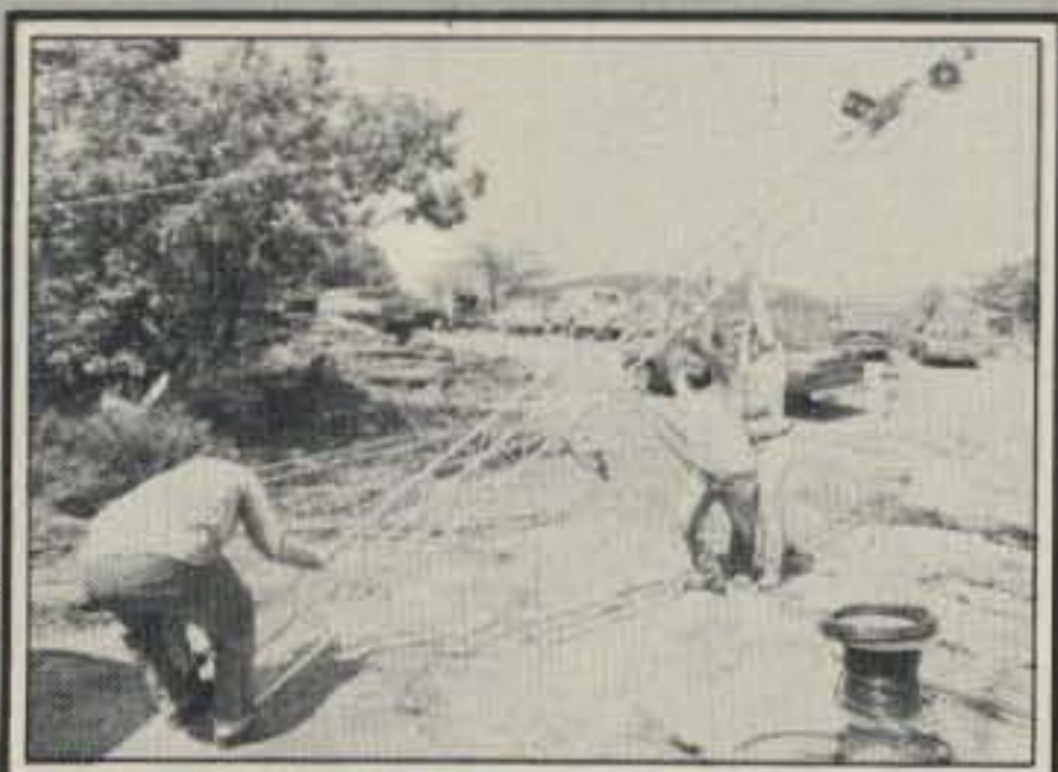
Hoisting the 1296 MHz tower are (left to right) W1HIV, WA1YLV, and K1PQO.
